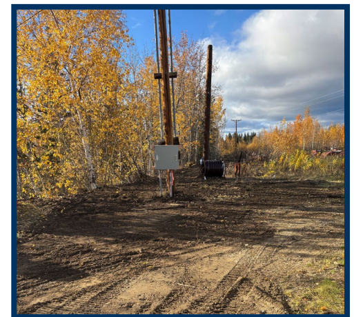
Fiber is being laid and made ready for service on the Northway Fiber project.
